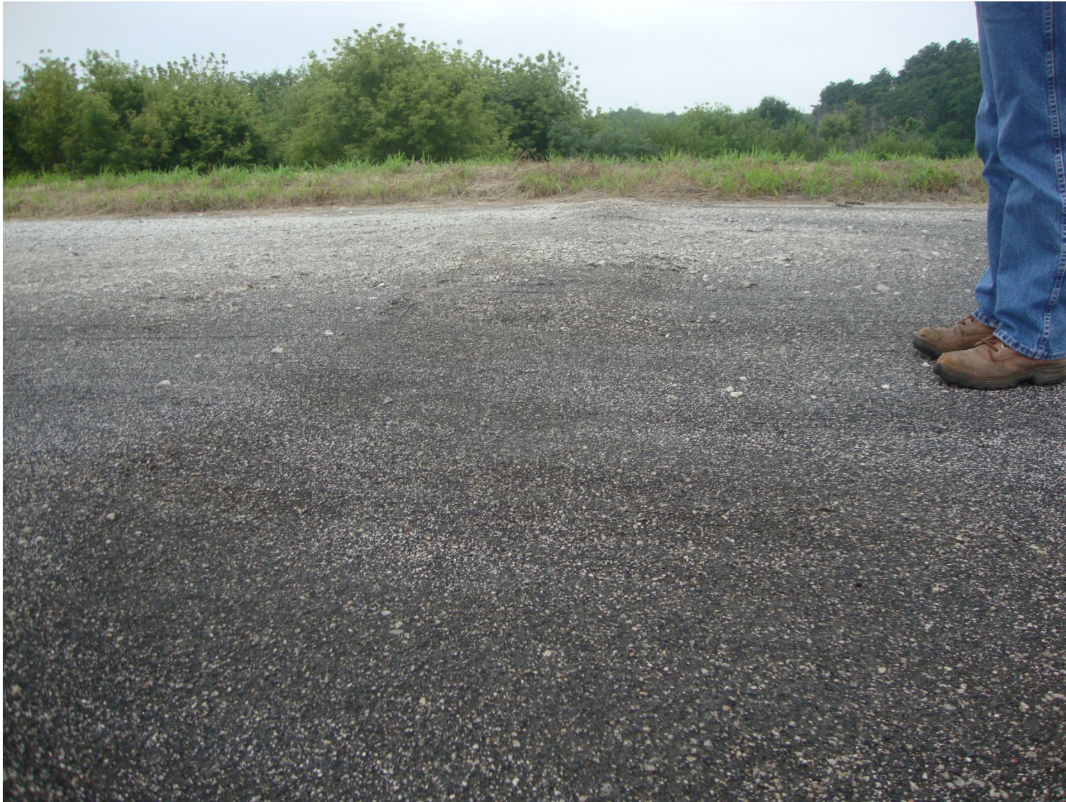
Compression heaving in crest of embankment
